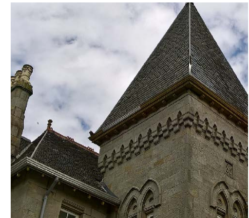
Roof flashing missing - Spanish slates in use
