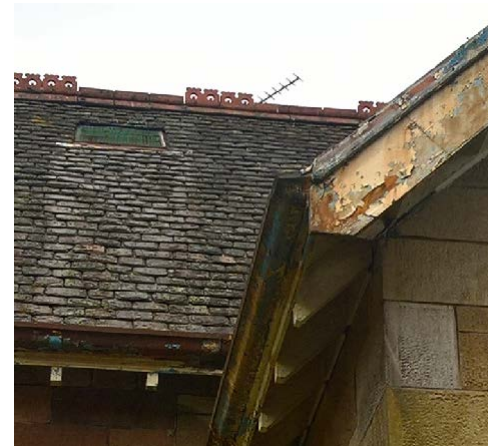
Blocked and corroded guttering
