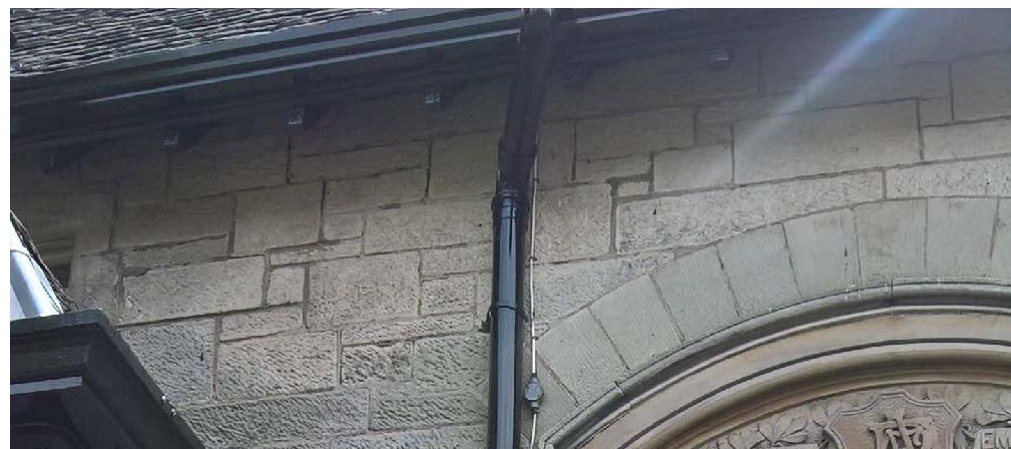
PVC downpipes in use
